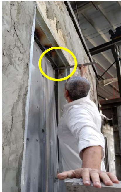
Figure 11: The observed movement after the hose stream.
